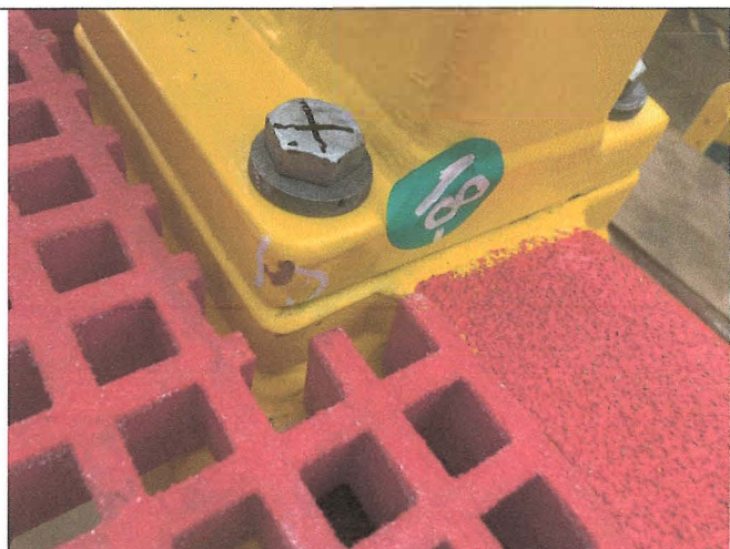
No. 18 - Mechanical damage.
