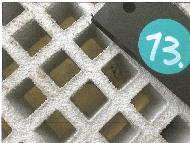
No. 13 - Dirt and fly rust under the gratings. Cleaning required.
