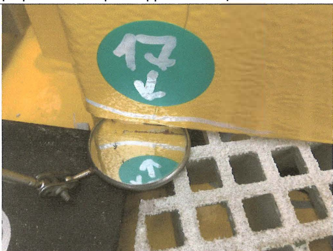
No. 17 – Kick plate edge, topcoat shall be removed, epoxy repair required.
