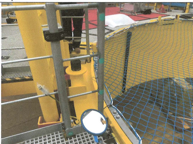
No. 15 – HDG handrails, not closed film, surface preparation and paint application required.
