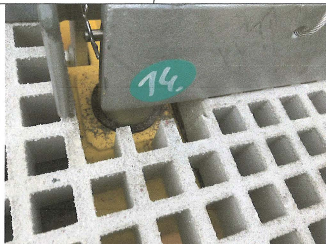
No. 14 - Dirt and fly rust under the gratings. Cleaning required.
